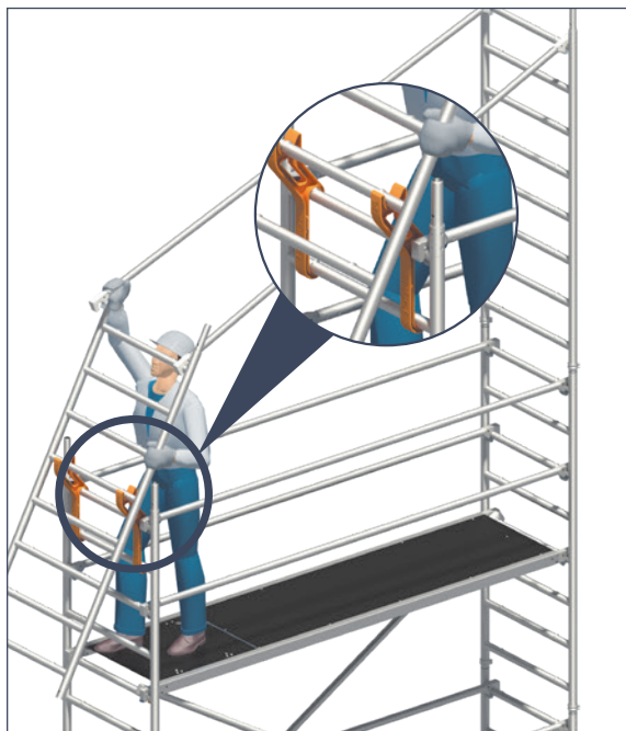
1 Fit the first ladder frame. Attach the Uni assembly hooks and position the second ladder frame for fitting of the rear guardrails.
